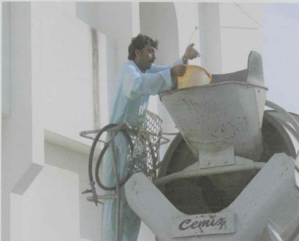
Figure 8: Wash water was added into the truck drum after unloading
